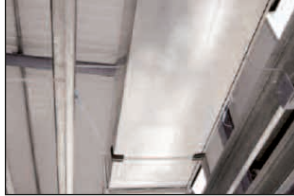
Square Air Ducts
